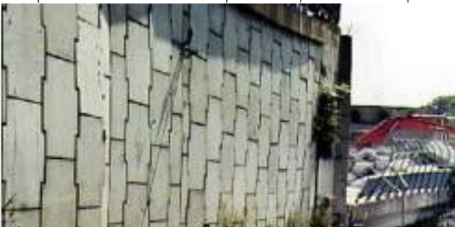
After the Izmit earthquake in 1999 - Turkey
